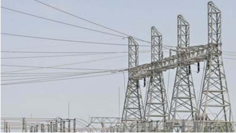
Power lines connect to an AES Ohio substation on Tipp-Cowlesville Road in Tipp City. Bryant Billing / Staff
